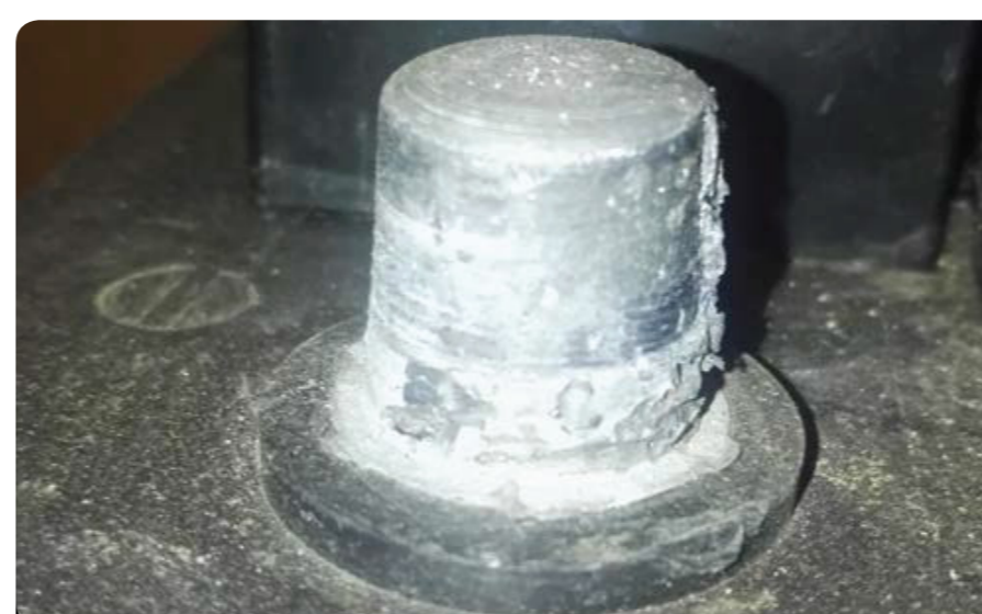
Terminal post damage caused from excessive force used when tightening post clamp.
