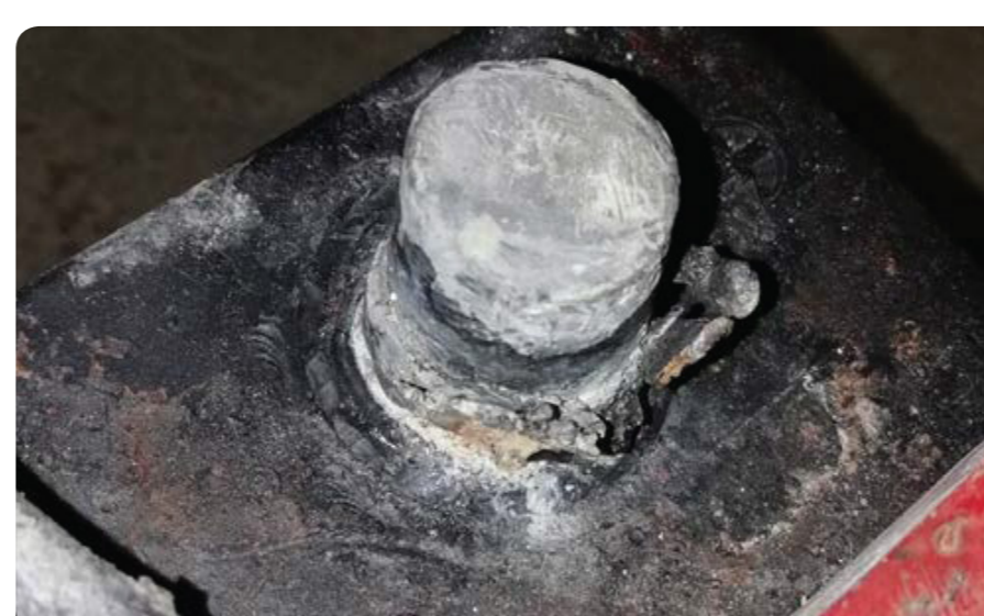
Damaged terminal post.
